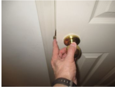
Basement closet door won't latch
