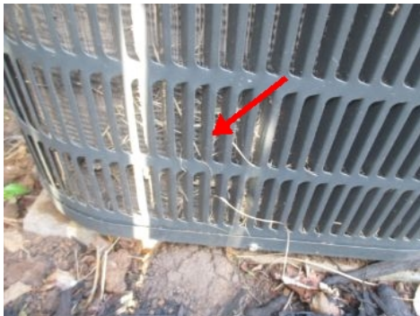
Clean grass from AC unit
