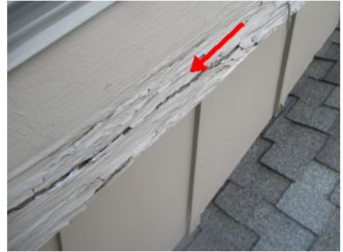
Damaged fascia board on roof
