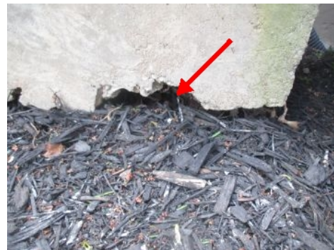
Small void under front porch
