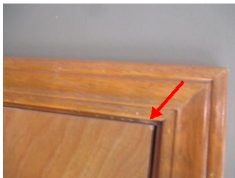
Hall door to master bedroom sticks at top
