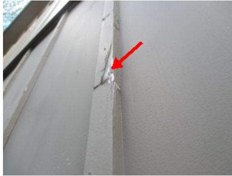
Flaking paint on right side of home
