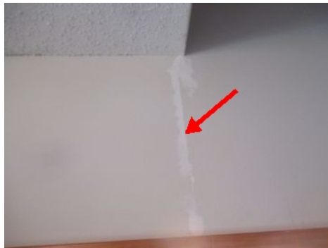
Drywall crack in hallway
