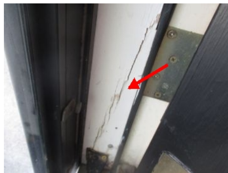
Damaged door jamb
