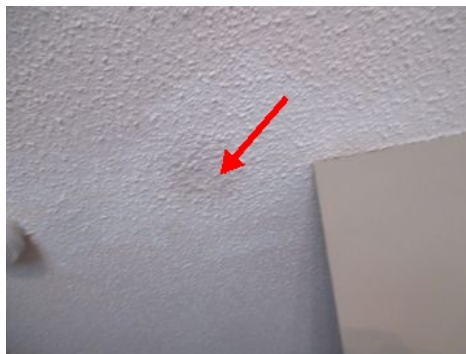
Water stain in hallway
