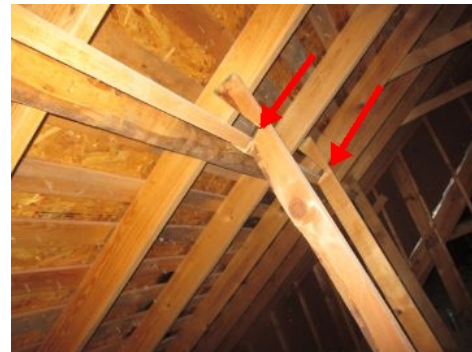
Roof braces miscut and loose
