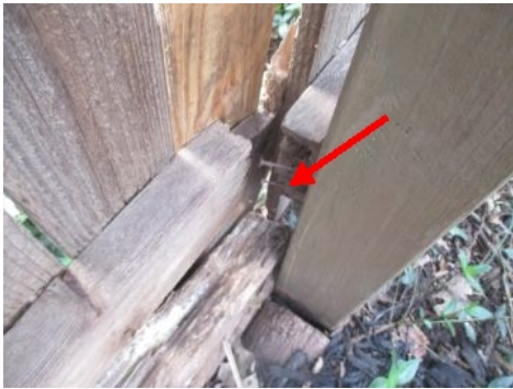
Damaged fencing at back side
