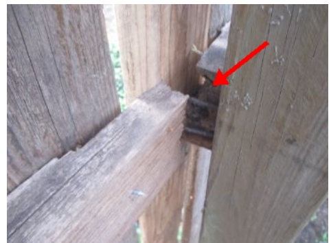
Damaged fencing at back side
