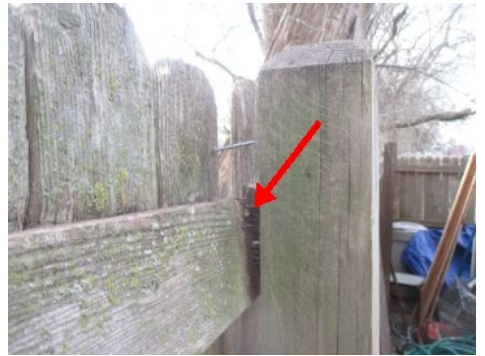
Damaged fencing at back side
