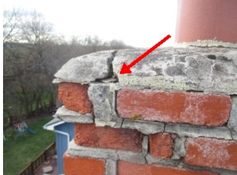
Damaged chimney cap
