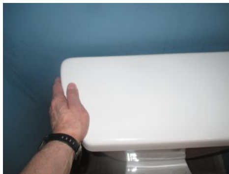
Loose tank in basement bath
