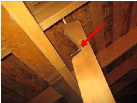
Roof braces miscut and loose
