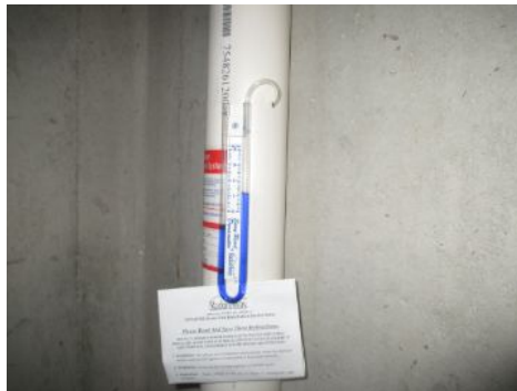
Radon vacuum monitor in basement
