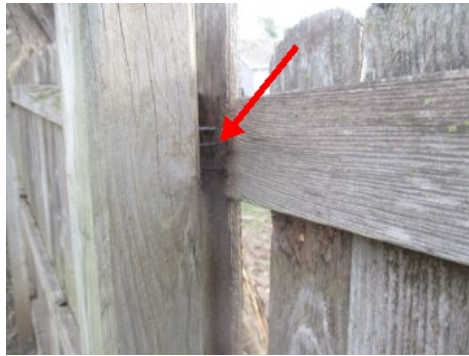
Damaged fencing at back side
