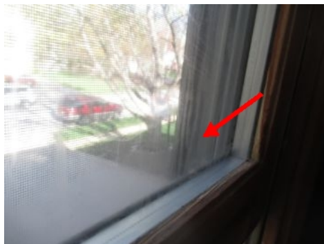
Window in middle front bedroom with broken seal
