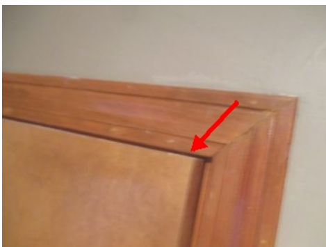
Bathroom door sticks at top
