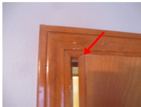
Hall door to middle front bedroom sticks at top
