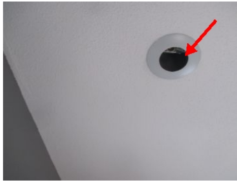
Missing light in middle back bedroom
