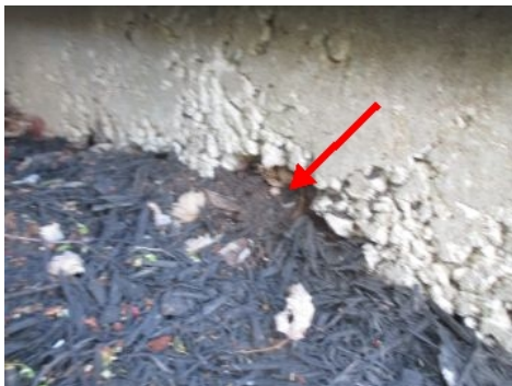
Small void under front porch
