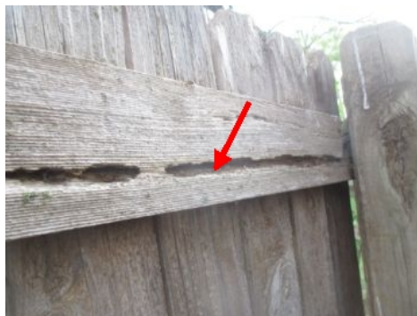
Damaged fencing at left side of yard
