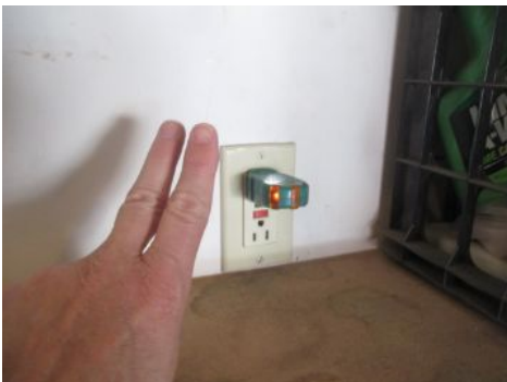
Bathroom GFIs reset in garage
